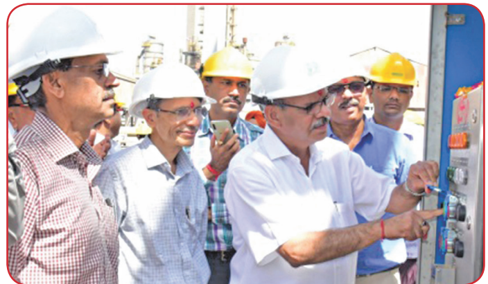
Installation and Commissioning of Motor Driven CO 2 Compressors at Hazira Plant (Surat)
